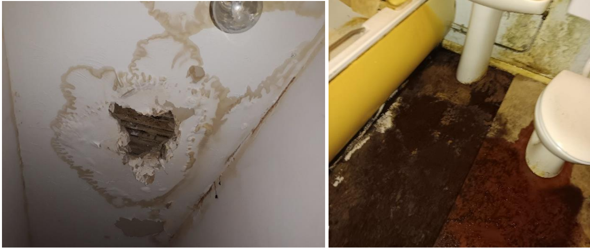
Traumatic damp caused by plumbing leaks.
