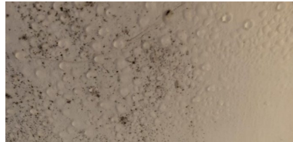
2 Ceiling condensation due to a lack of surface warmth, insufficient air change or both
