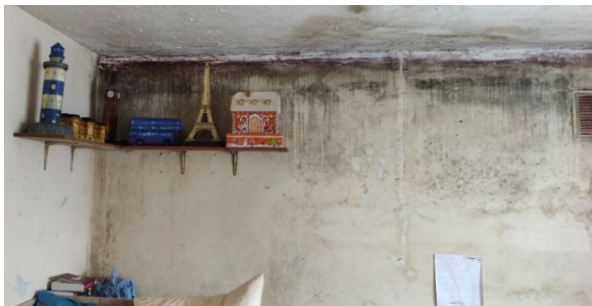
1 Mould formation on the coldest surfaces
